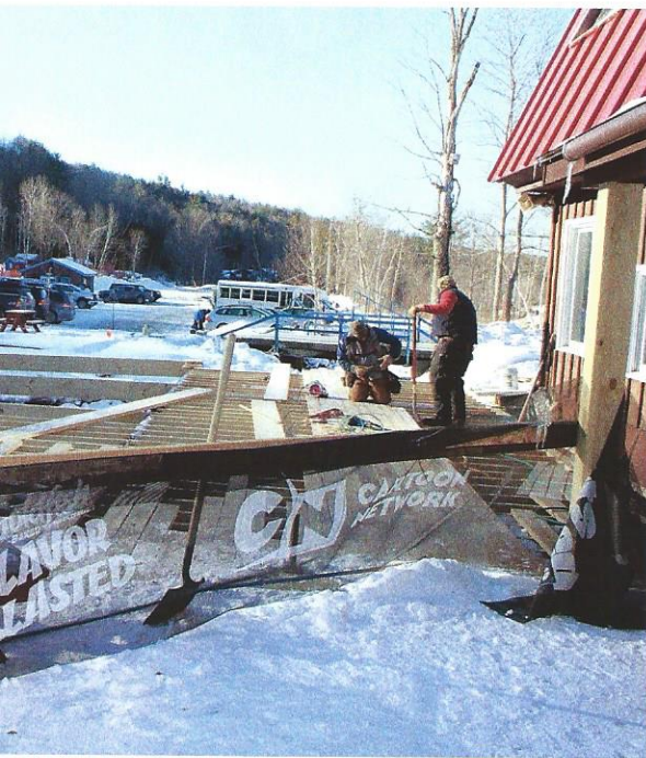
Opposite top: A volunteer repaints Whaleback Mountain's base lodge. Opposite bottom and above: Whaleback's deck gets much-needed repairs after damage by Tropical Storm Irene.
